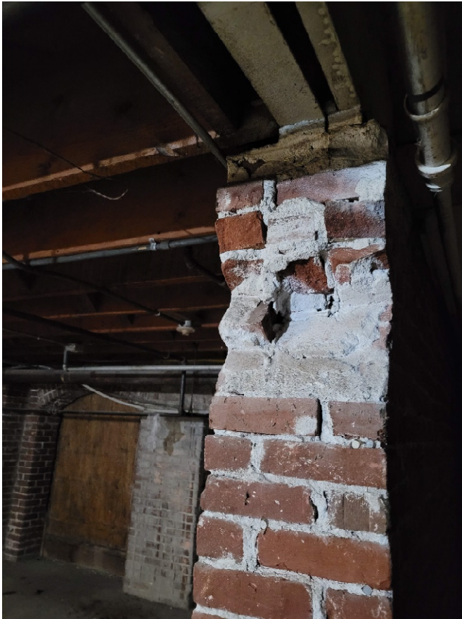
Photo of damage looking to the east.
