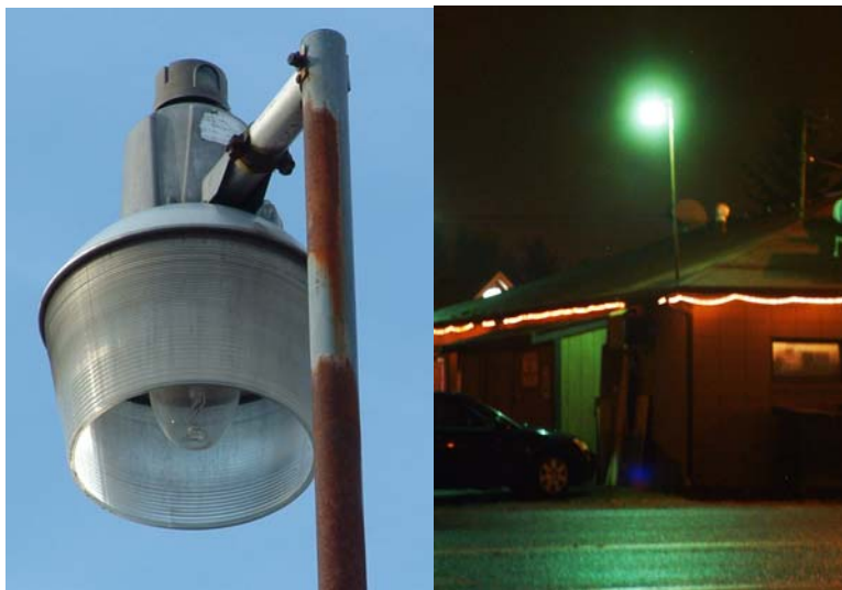
Unshielded yard blaster light at Point Tavern
