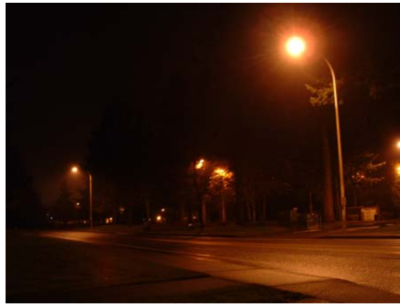
High pressure sodium (New Market Streetlights)
