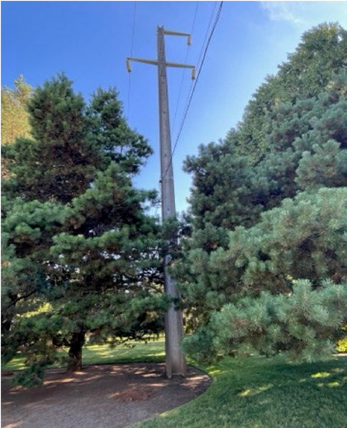
Transmission Tower Example in Southcliff
