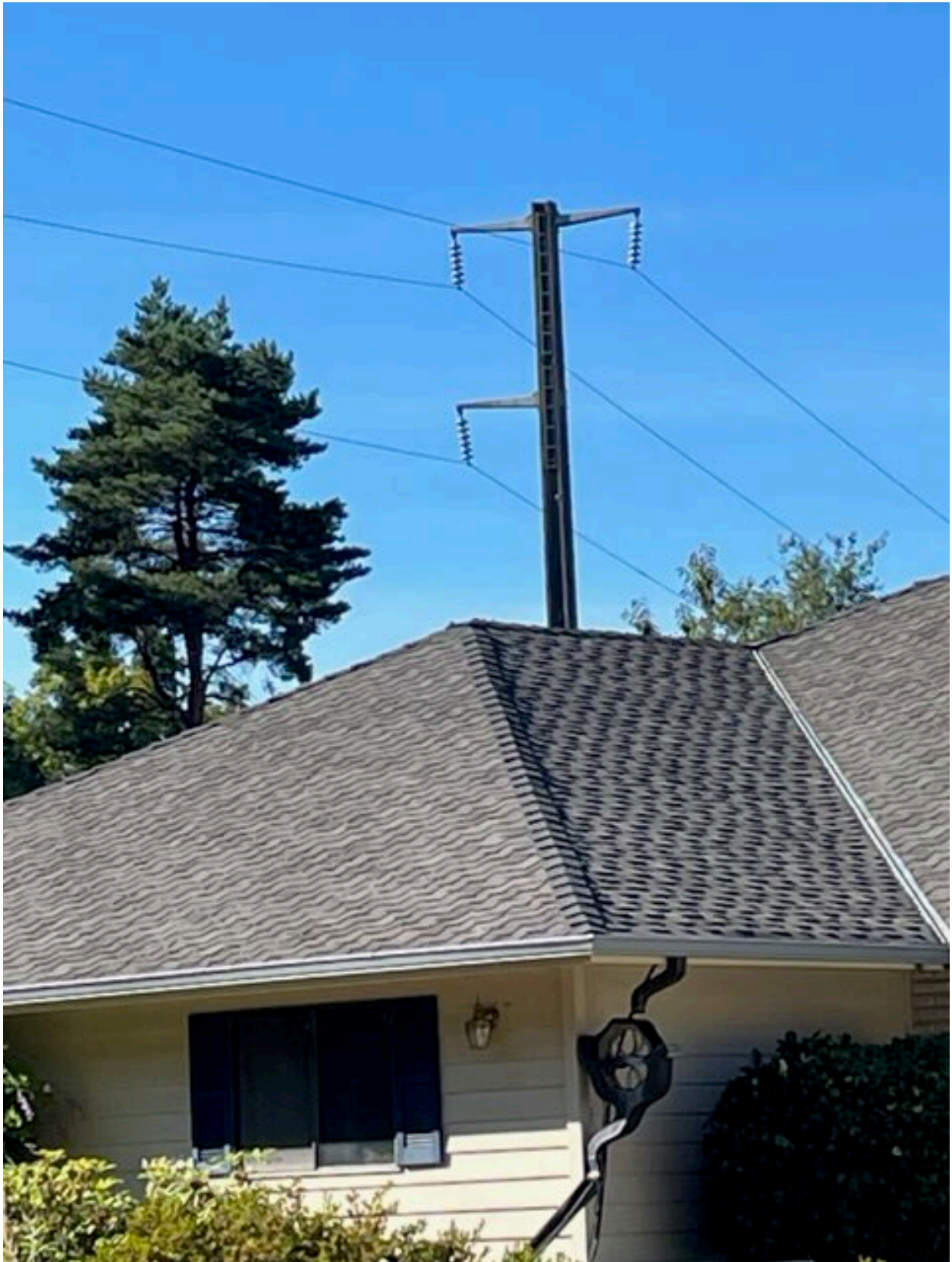
Transmission Tower Between Oregon Drive and Mill Plain Boulevard
