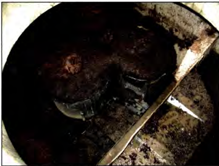
Media Cartridge Filter Vault with Accumulated Sediment
