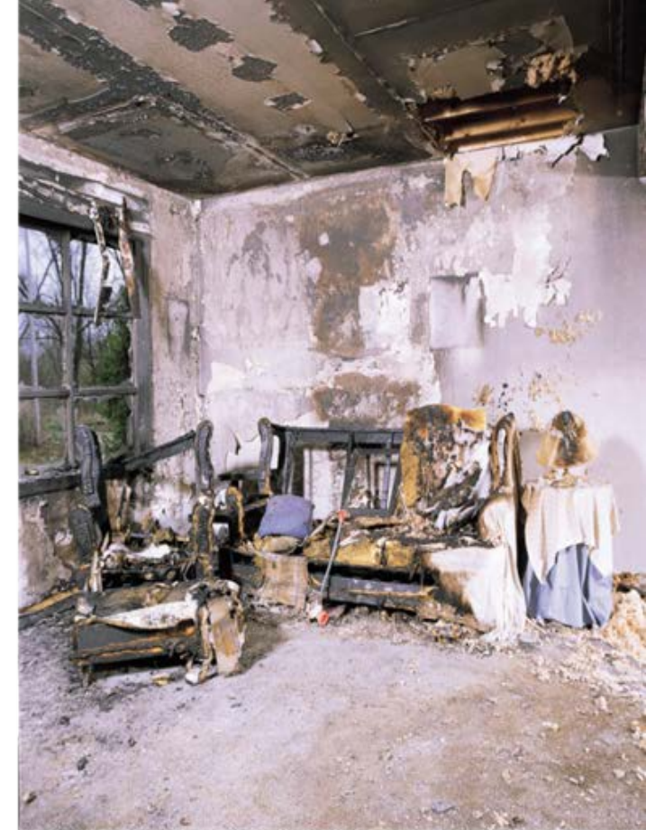
Damage without fire sprinklers
